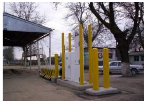
Typical vehicle monitor installation
