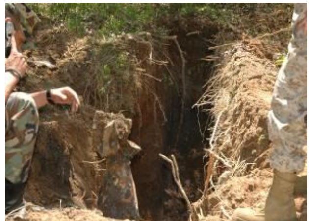
UXO Encountered in Test Pit Excavation
