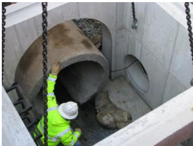
Aligning Doghouse Enclosure
