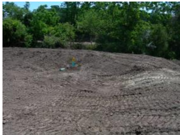
Low Level Dike and Water Level Standpipe
