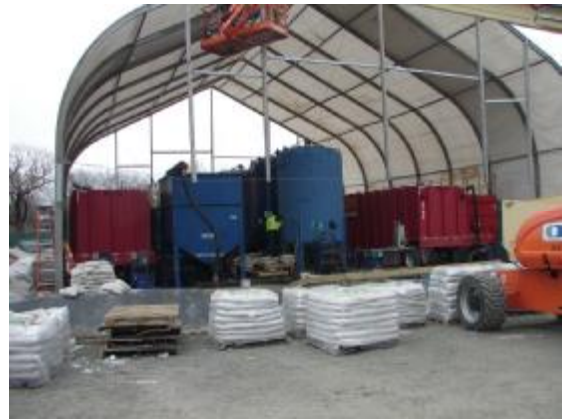
Water Treatment System
